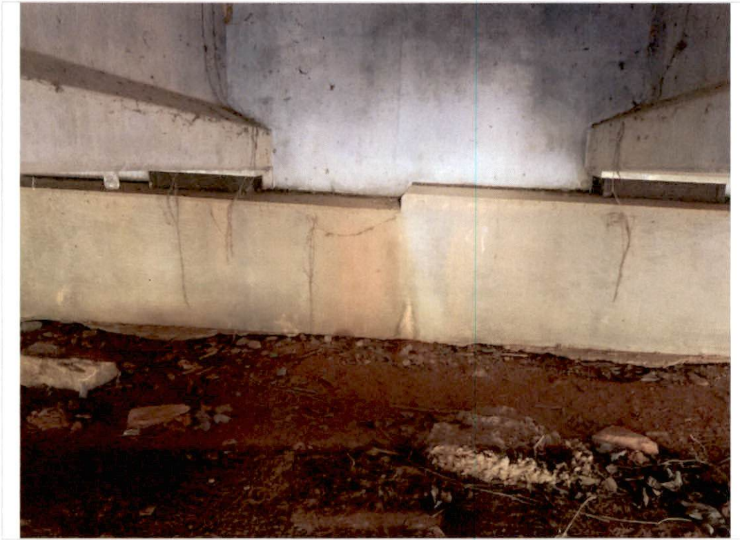
Abutment 1 cap, minor vertical cracking. 2024
