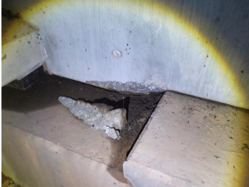
Photo 11 - Spall in End Bent 1 Curtain Wall near Beam 6 and cap step
