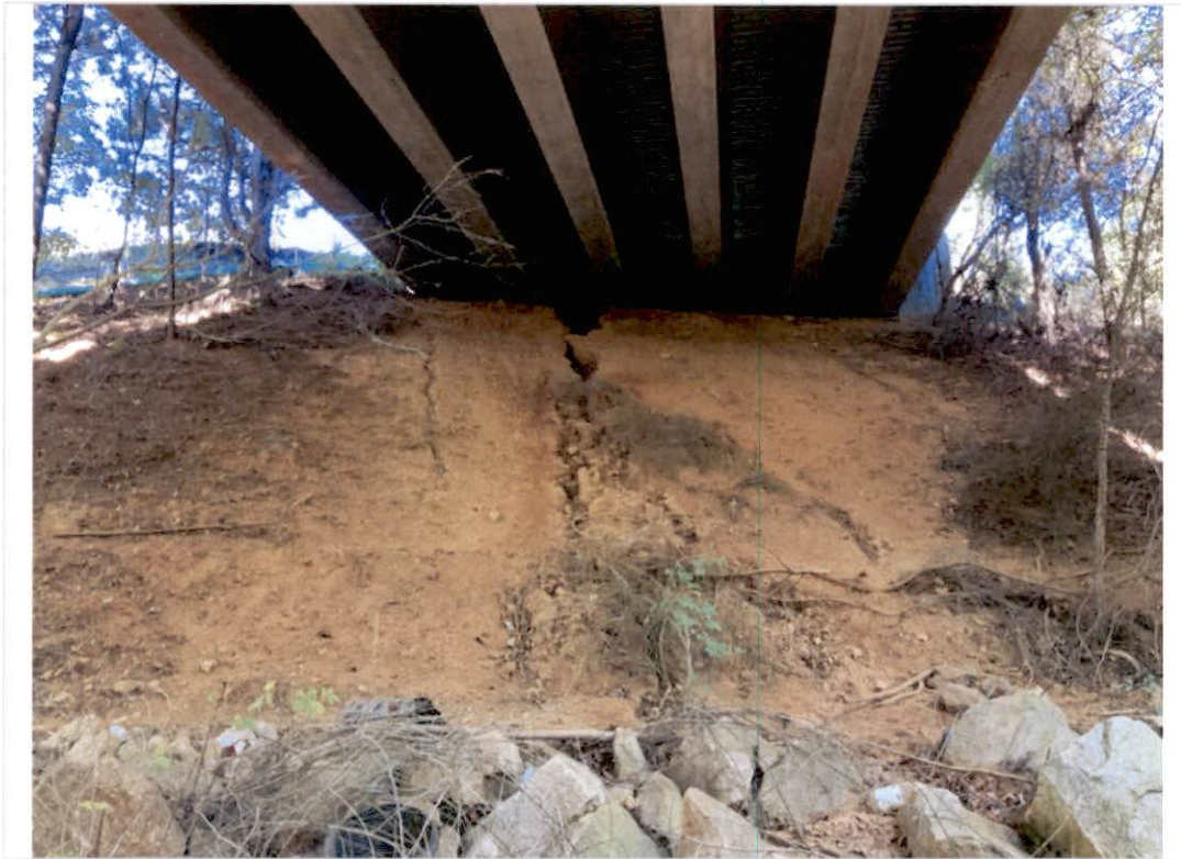
Abutment 4 slope erosion. 2024
