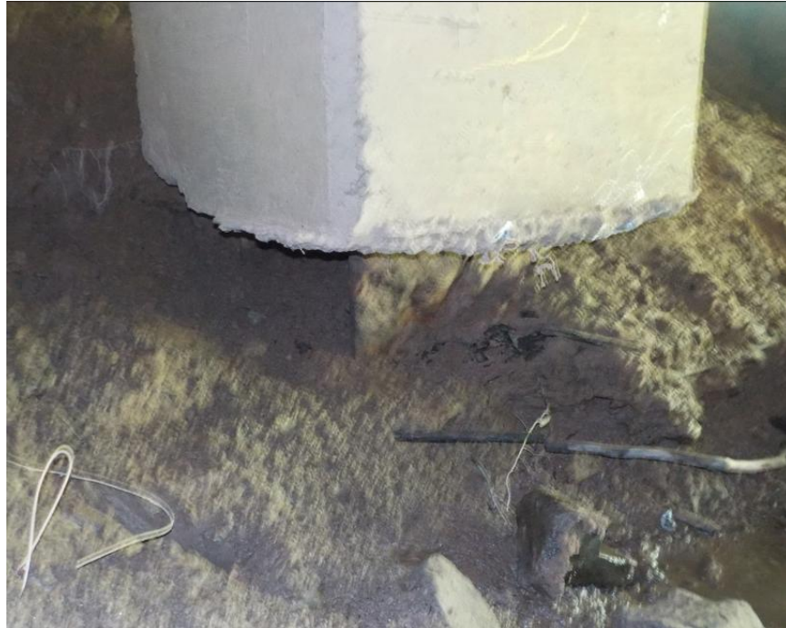
Photo 18 - Bent 3, Pile 4 with 10" exposed steel pile with minor corrosion
