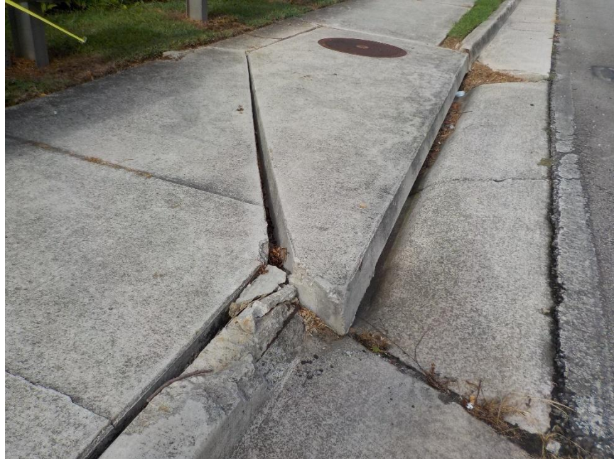
Photo 32 - Rear approach slab (at End Bent 1) spalled curb 2'-0" L x 6" W x 5" H and catch basin lid displaced.
