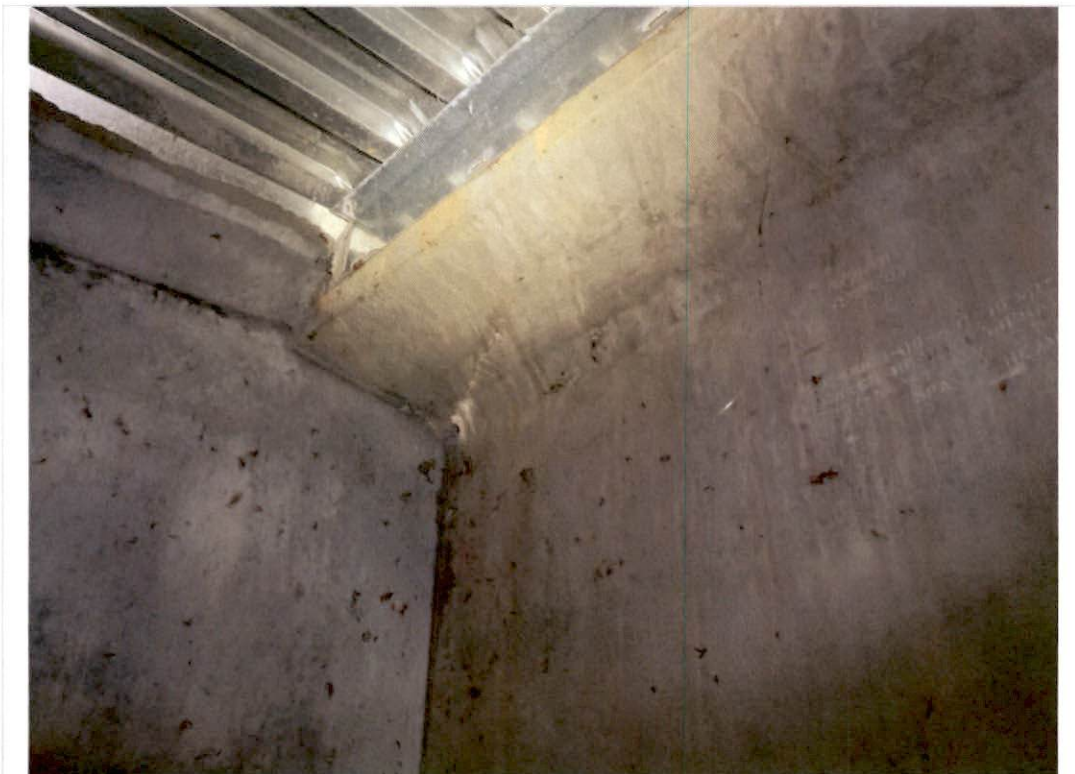
Span 1 rear, beam m 3, top right flange. Hairline crack with efflorescence. 2024
