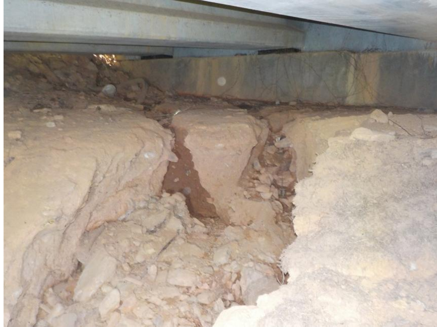
Photo 7 - Erosion of slope underneath of End Bent 4 (Closeup of berm area)
