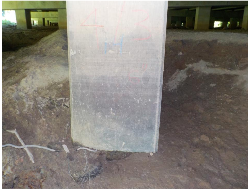
Photo 22 - Bent 4, Pile 3 with 6" exposed steel pile with minor corrosion
