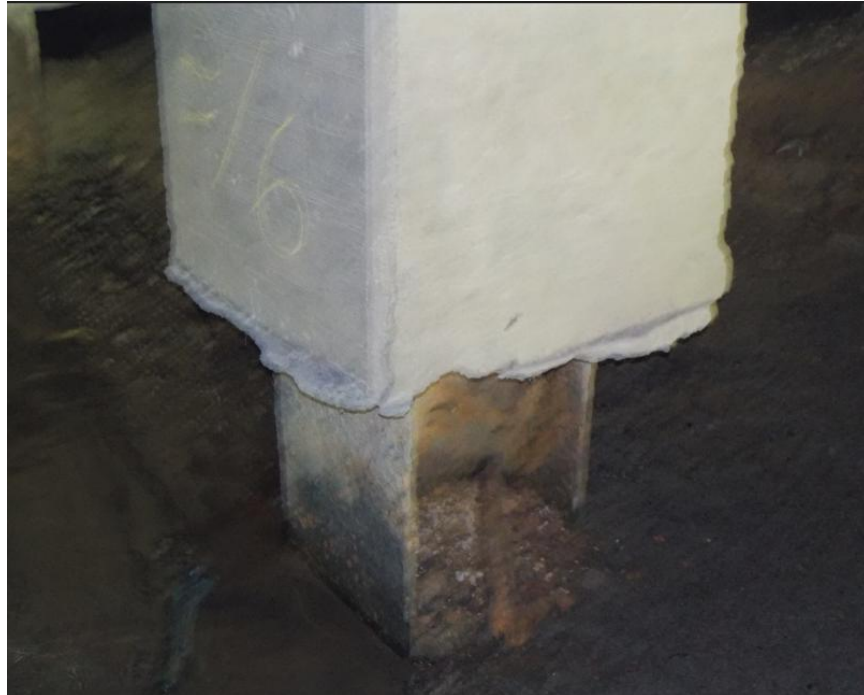
Photo 20 - Bent 3, Pile 6 with 2'-0" exposed steel pile with minor corrosion
