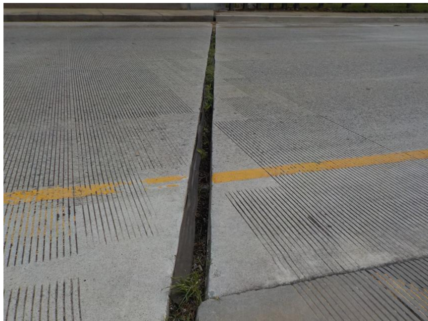
Photo 15 - End Bent 10, up to 3 ½" width. The joint material has failed.
