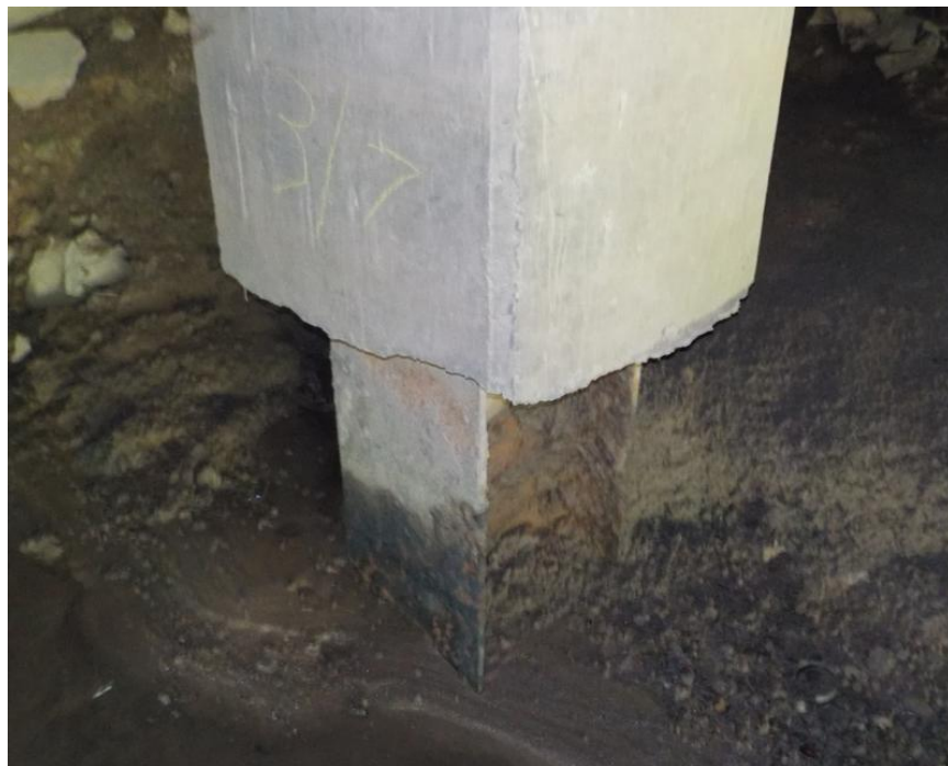
Photo 21 - Bent 3, Pile 7 with 2'-0" exposed steel pile with minor corrosion
