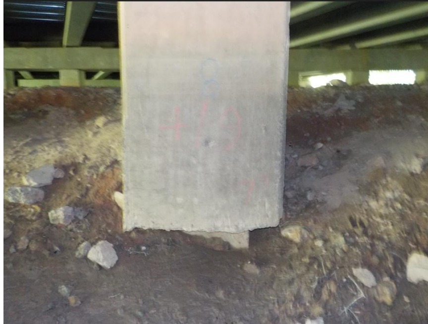
Photo 28 - Bent 4, Pile 9 with 7" exposed steel pile
