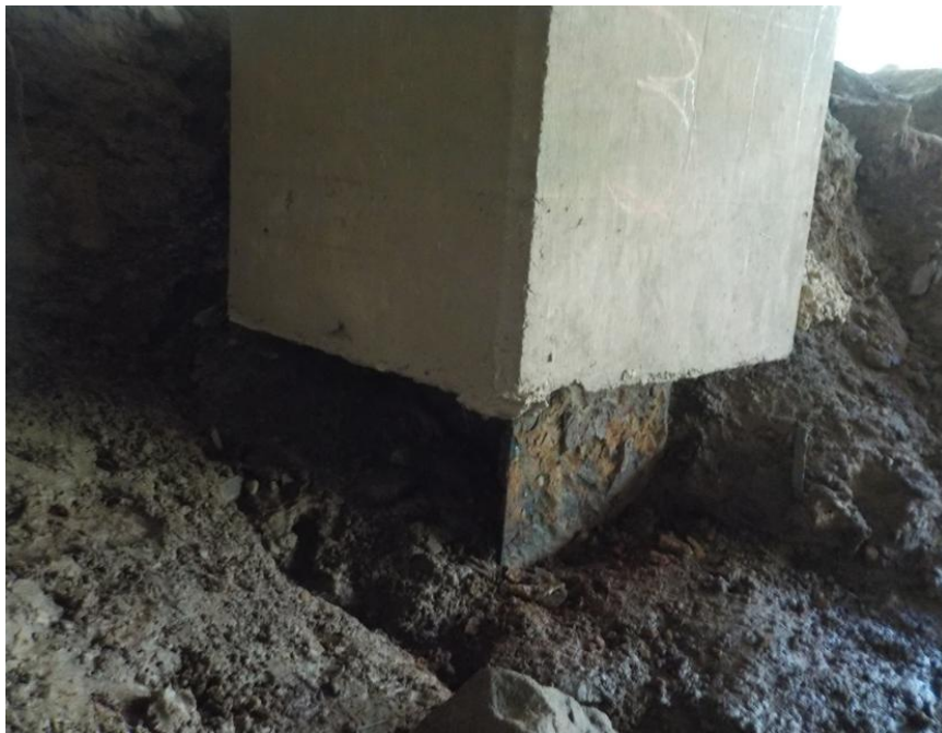
Photo 17 - Bent 3, Pile 3 with 1'-0" exposed steel pile with minor corrosion
