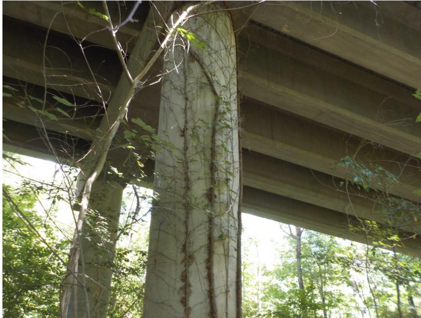
Photo 9 - Vegetation growth at Column 1 Bent 3, other columns are similar
