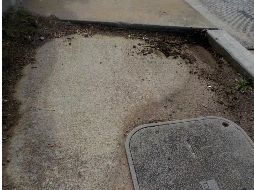
Photo 34 - Sidewalk has settled up to 5" for 12'-0" L x 5'-6" W (north west corner)
