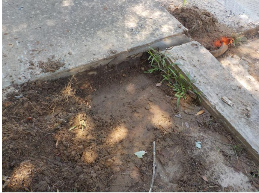
Photo 3 - Sidewalk settlement of approximately 5 ½" (4'-10" L x 5'-3" W x 5 ½" H)
