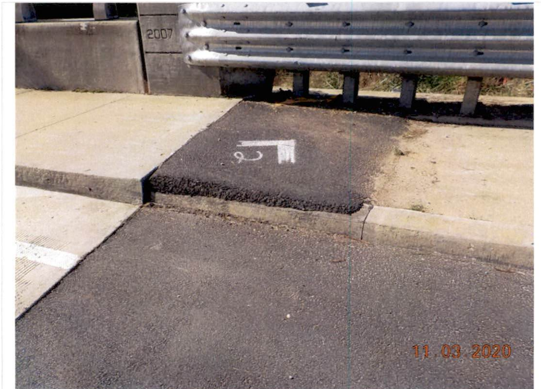
Forward left sidewalk has cracked, settled. Repaired 2020
