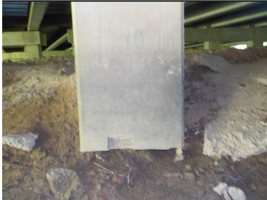
Photo 26 - Bent 4, Pile 7 with 4" exposed steel pile
