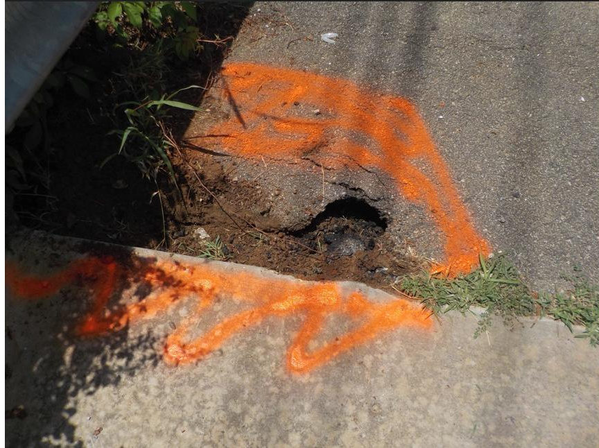
Photo 5 - Sidewalk repair required at northwest corner (1'-3" L x 3' W x 7" H)
