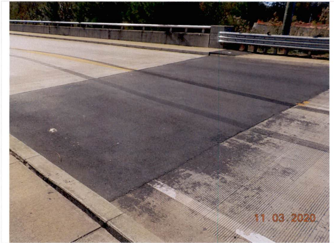
Forward approach slab settlement repaired. 2020 See 2024 new settlement photo.
