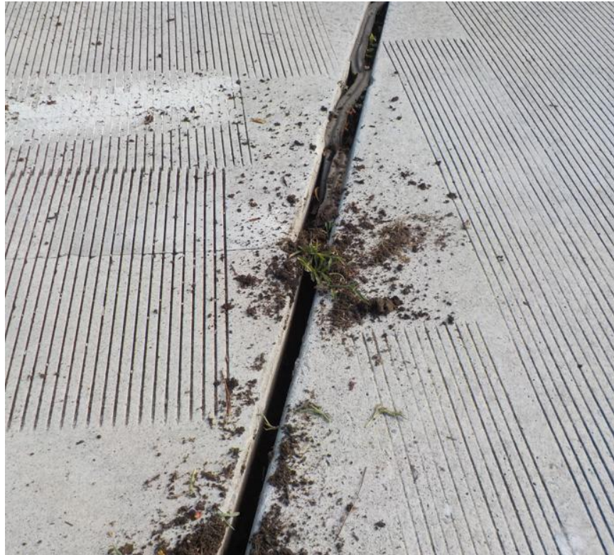
Photo 12 - End Bent 1, west bound lane missing and broken joint material (close view)
