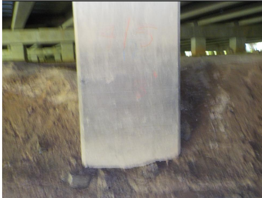
Photo 24 - Bent 4, Pile 5 with 3" exposed steel pile with minor corrosion
