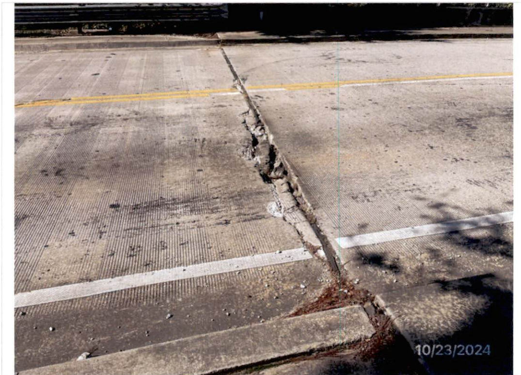
Rear approach slab settlement up to 2.0" causing moderate spalling up to 12.0' long x 14.0" wide x 6.0" deep in the northbound travel lanes at abutment 1. 2024
