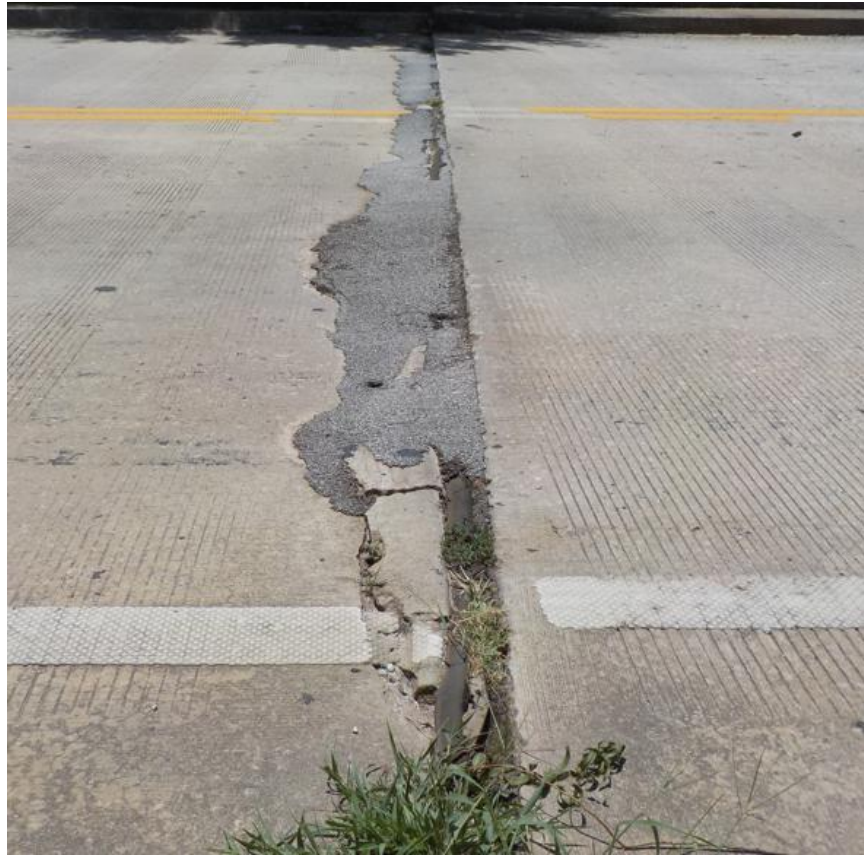
Photo 1 - Spalling at Rear Approach Slab (at End Bent 1)
