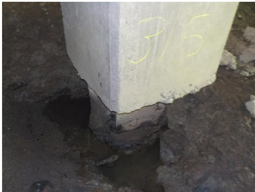
Photo 19 - Bent 3, Pile 5 with 2'-0" exposed steel pile with minor corrosion
