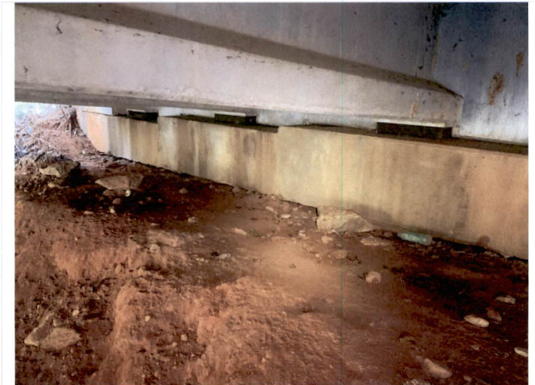
Abutment 1, right side underneath area of approach slab settlement. 2024
