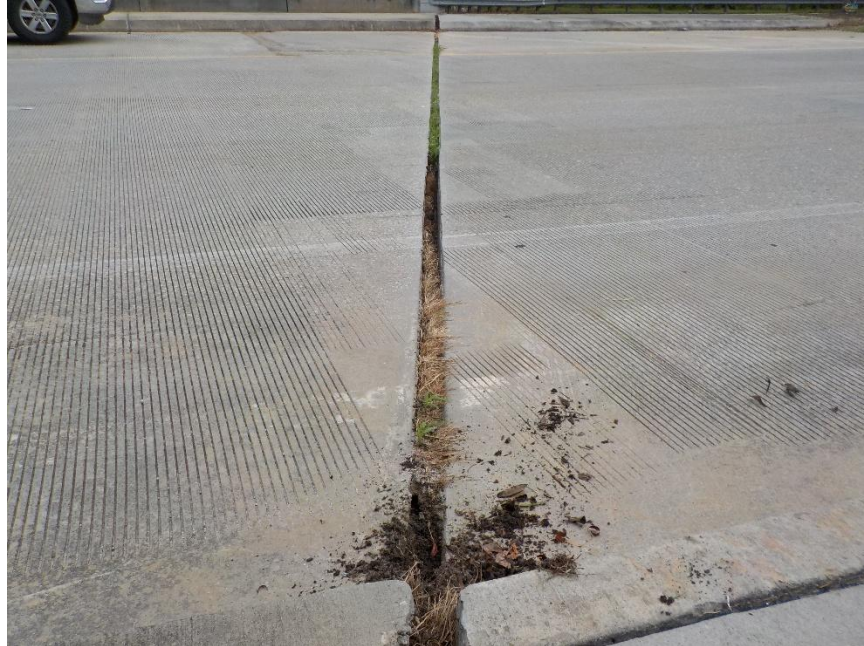
Photo 14 - End Bent 10 Joint, width varies from 2 ¾" and 3 ½" filled with debris. Joint material loose or missing
