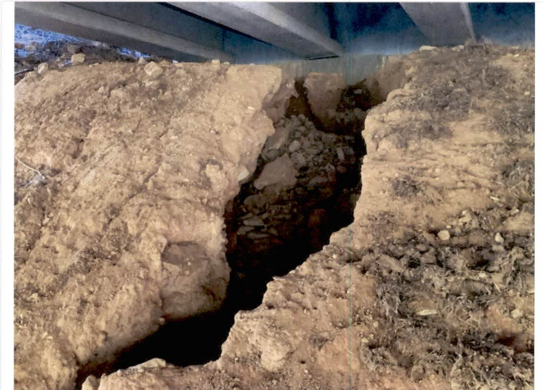
Abutment 4 slope erosion. 2024 Close up
