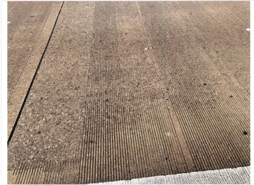
Typical transverse cracking in the deck top.
