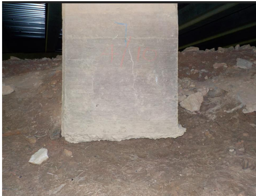
Photo 29 - Bent 4, Pile 10 with 4" exposed steel pile
