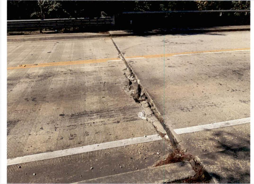
Rear approach slab settlement with moderate spalling. 2024.
