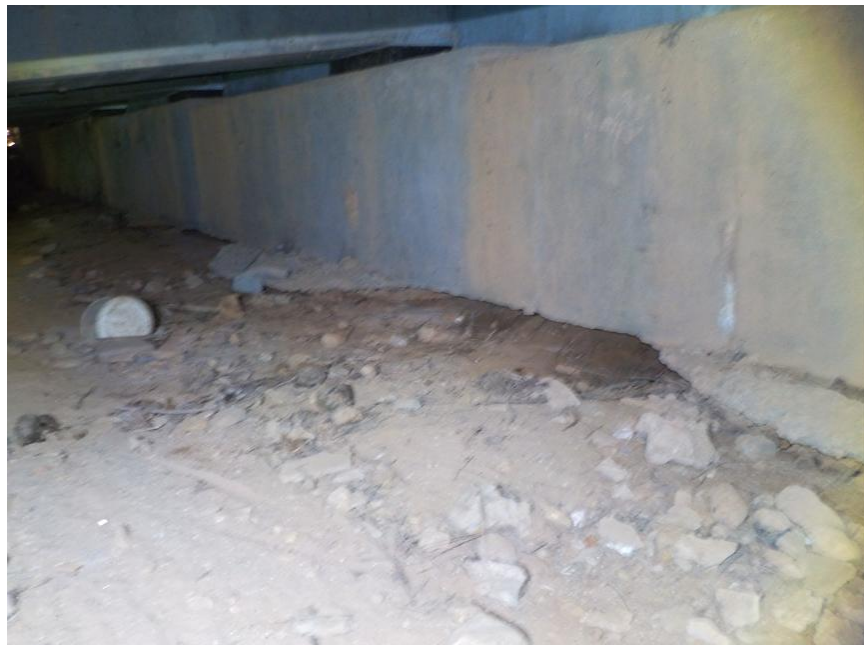
Photo 6 - Erosion underneath End Bent 4 cap (3'-4" L x 24' W x 3" H)
