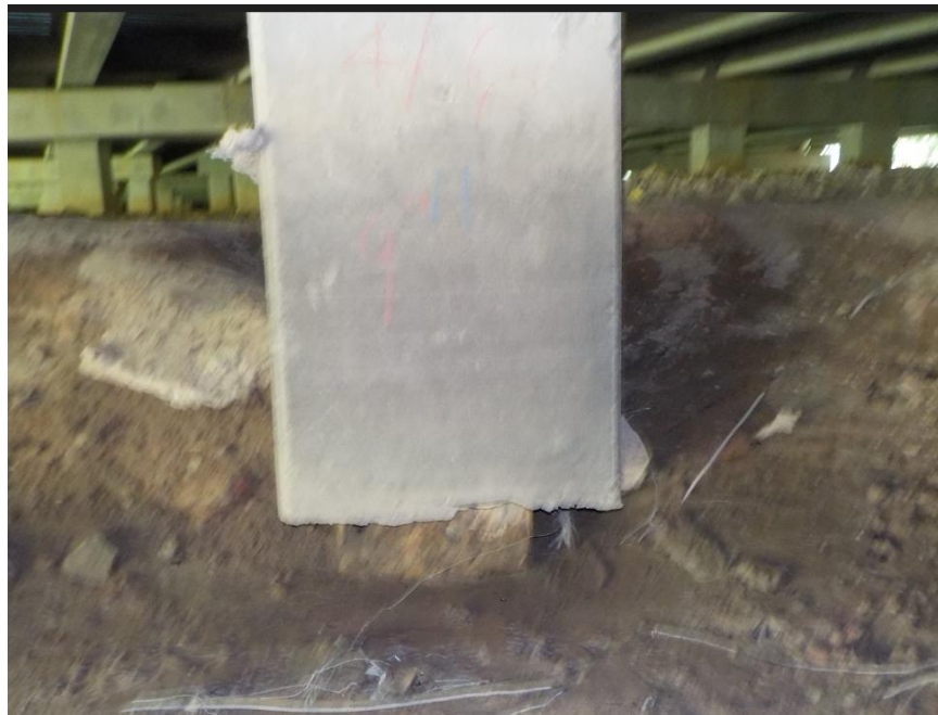
Photo 25 - Bent 4, Pile 6 with 9" exposed steel pile with minor corrosion
