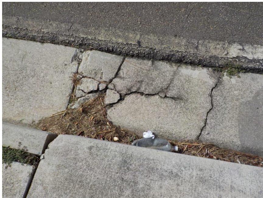
Photo 33 - Gutter cracking 3'-0" L x 2'-0" W at the northeast corner.
