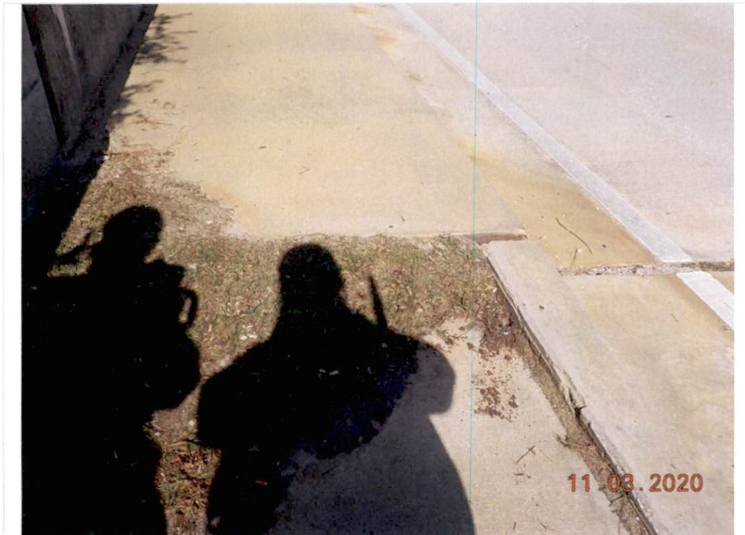
Rear left sidewalk settlement
