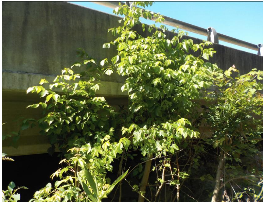
Photo 31 - Trees growing into the bridge
