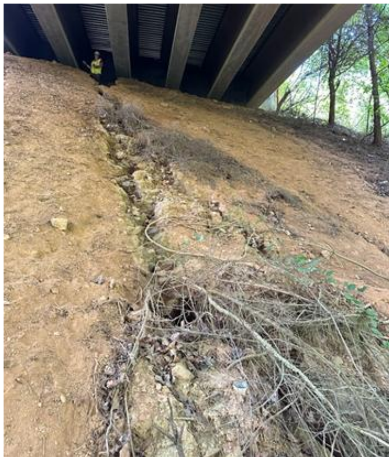
Photo 8 - Erosion of slope underneath of End Bent 4 (60' -0" L x 6' -0" W x 2'-0" H)
