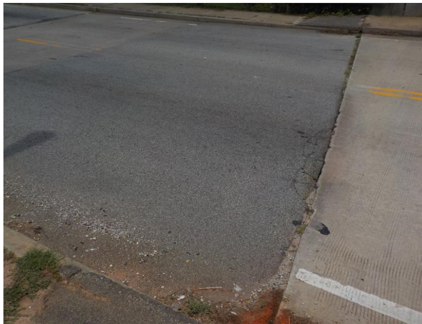
Photo 2 - Forward Approach Slab 2" Settlement at End Bent 4
