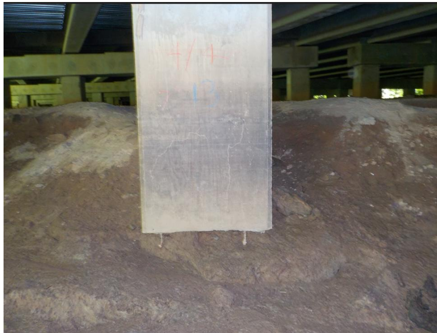
Photo 23 - Bent 4, Pile 4 with 7" exposed steel pile with minor corrosion
