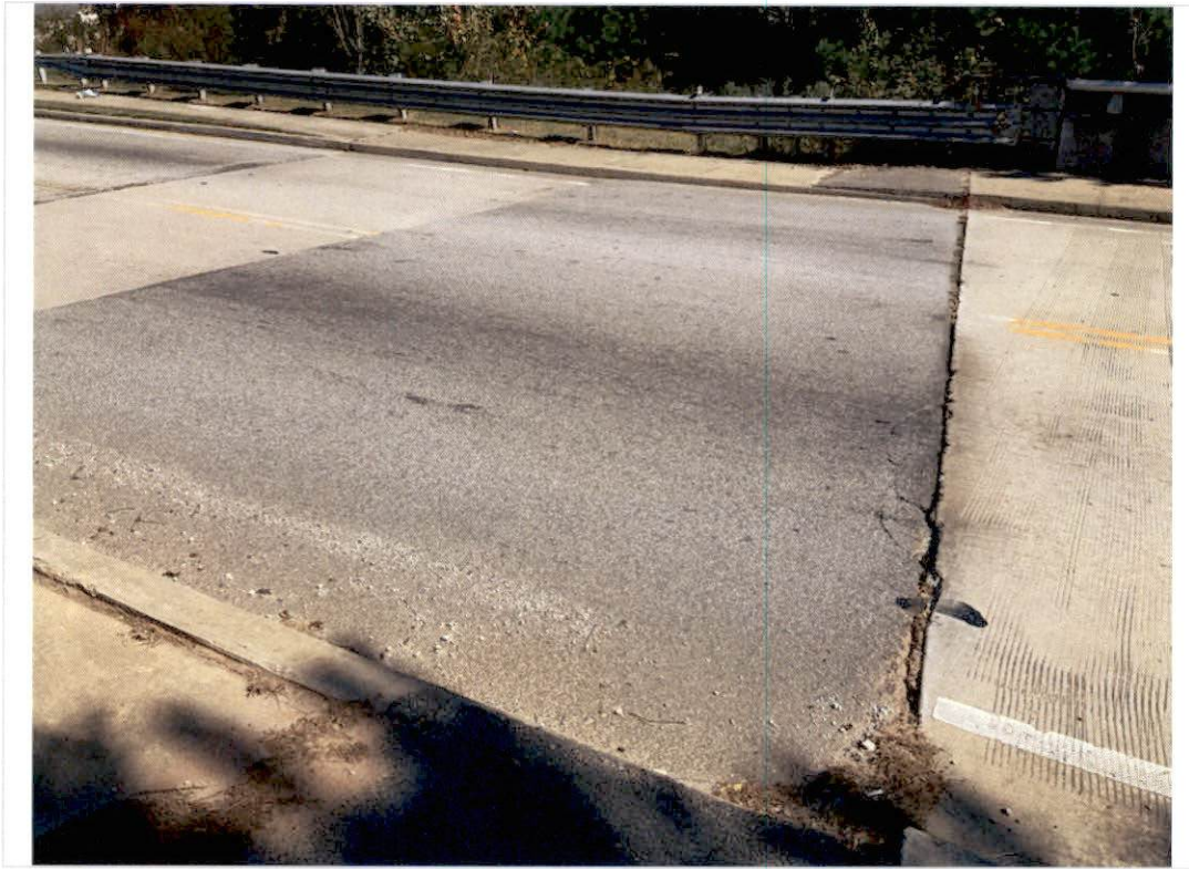
Forward approach slab, new settlement up to 1.0". 2024
