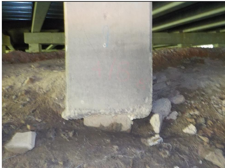
Photo 27 - Bent 4, Pile 8 with 8" exposed steel pile
