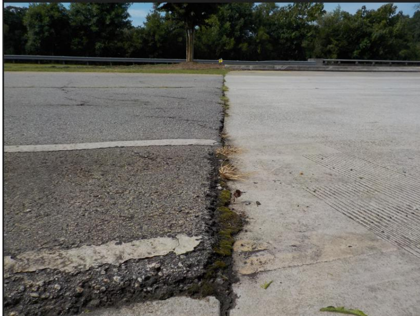
Photo 16 - Asphalt heaving up to 2" at transition between roadway and approach slab
