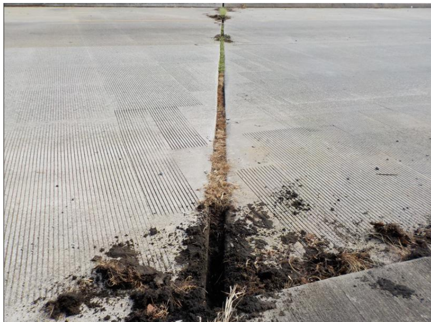
Photo 13 - End Bent 1 Joint, up to 3" width and filled with debris and joint material loose in travel lanes and missing at shoulder
