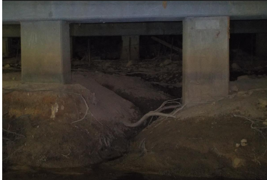
Photo 30 - Bent 3, Erosion channel between piles 14 and 15
