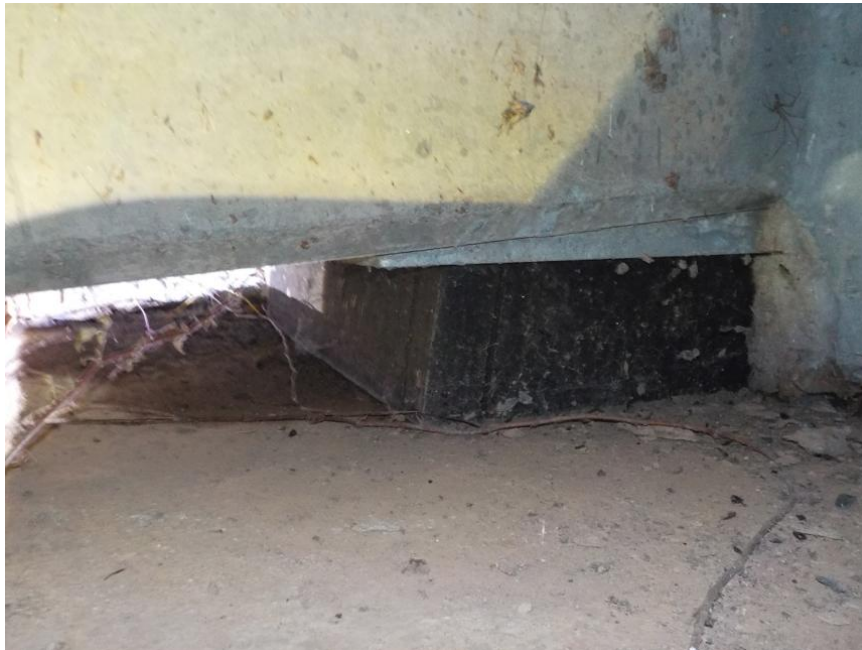
Photo 10 - Bearing pad under Girder 1 at End Bent 4. (Expanded up to \frac{3}{4} " at the top. Other girders at End Bent 4 are expanded up to \frac{1}{4} " )
