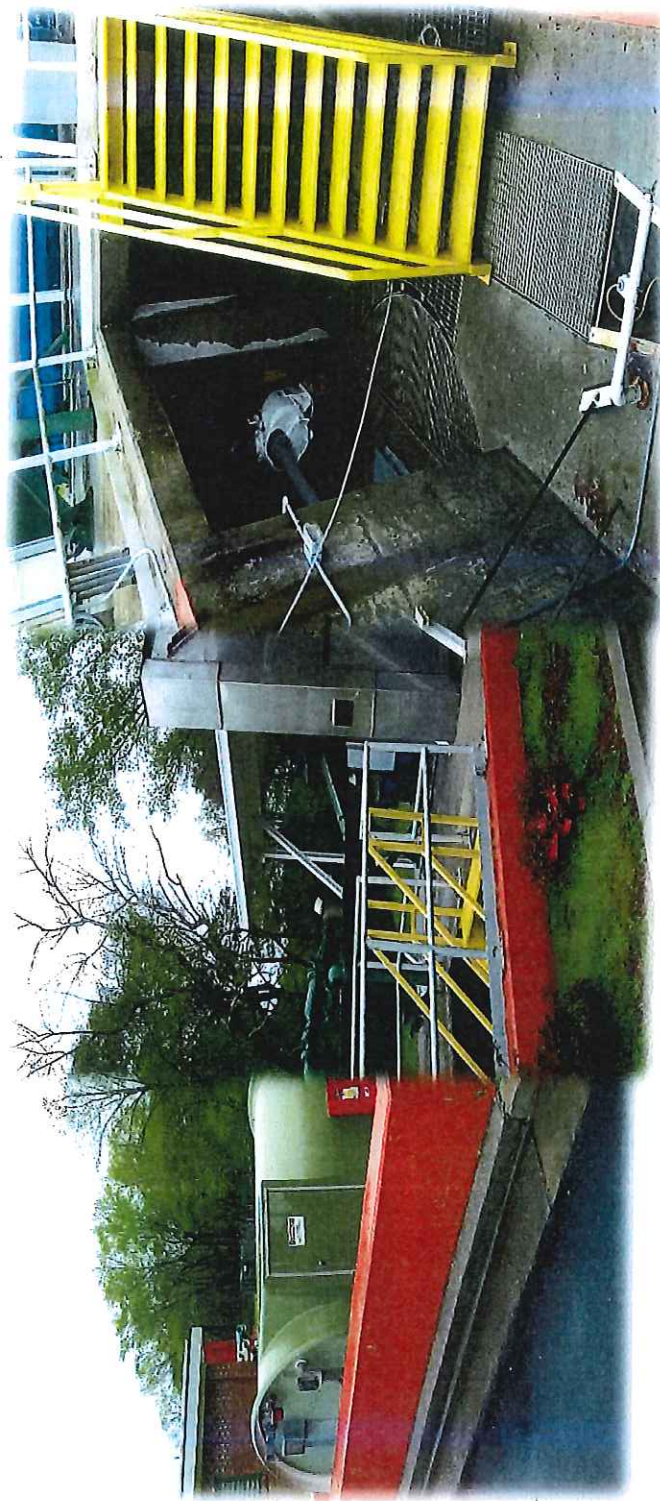
Headworks Main Pumping Station
