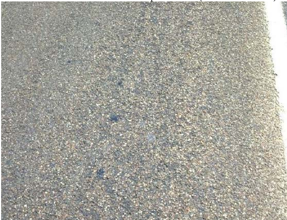
Level 1 – loss of substantial number of stones
