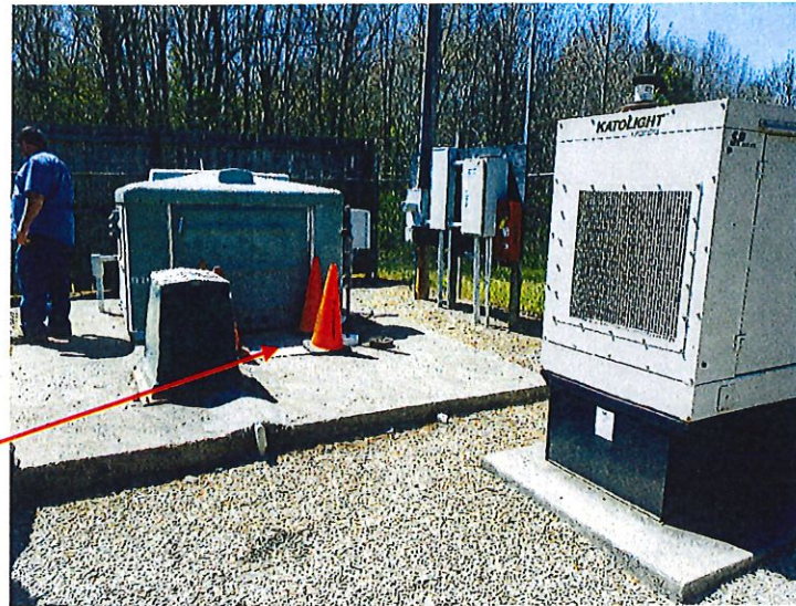
Figure 3: Old Conyers Lift Station
