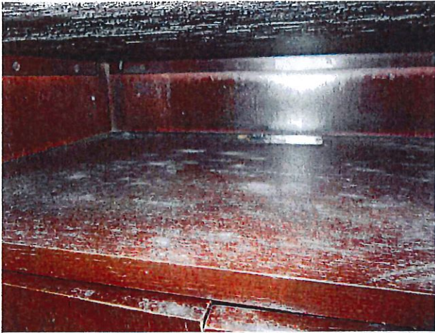
7. View of suspect mold growth on furniture within the Court Room (Municipal Court Building).
