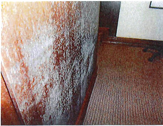
5. View of suspect mold growth on furniture within the Court Room (Municipal Court Building).
